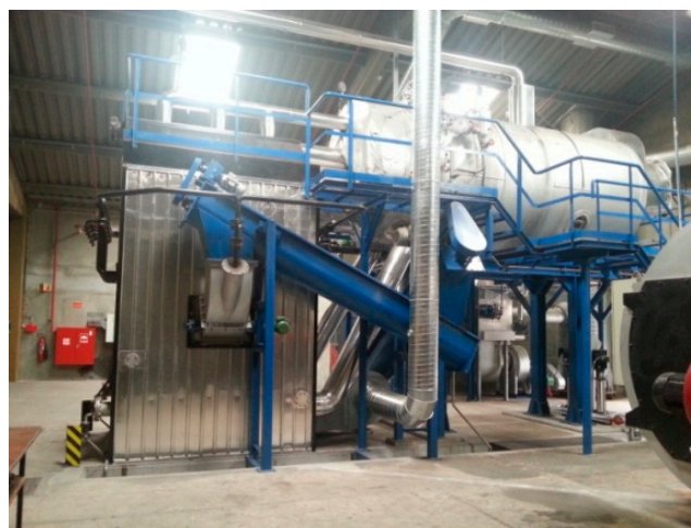
Figure 7. Example of a biomass burner in a steam boiler of a textile production plant.
