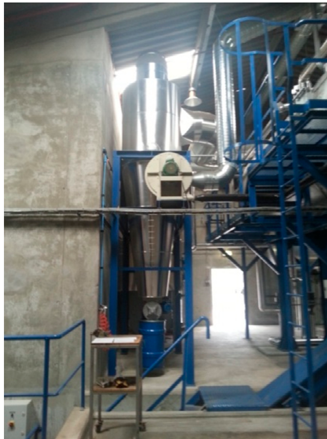
Figure 9. Biomass steam boiler filtering system.
