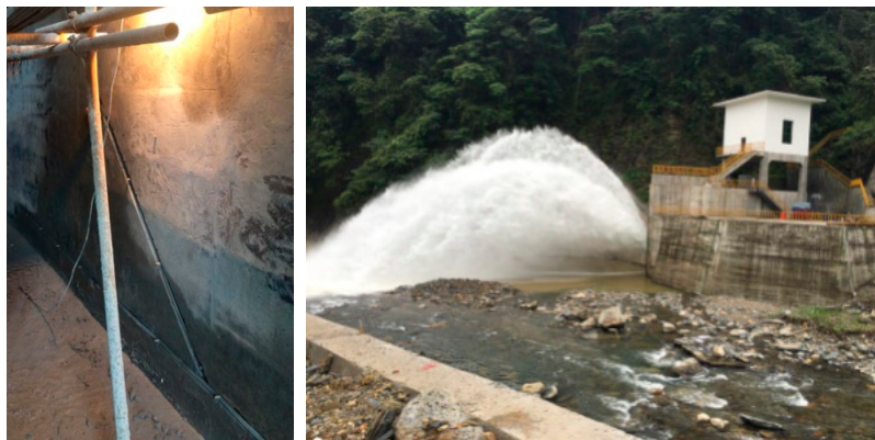
Figure 22. Engineering application of the polyurea-based coating for the flood discharge tunnel of the Daotang Reservoir.
