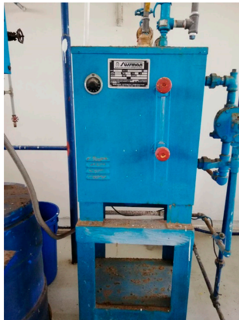
Figure 5. Liquefied petroleum gas (LPG) boiler used for steam production.
