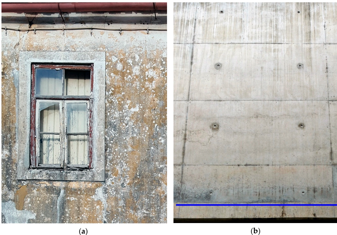
Figure 4. Examples of causes of defects: (a) degradation due to natural ageing in a window frame, a natural stone jamb and a wall render in a vacant house; (b) a deficient architectural concrete surface due to a badly executed casting/panel joint.
