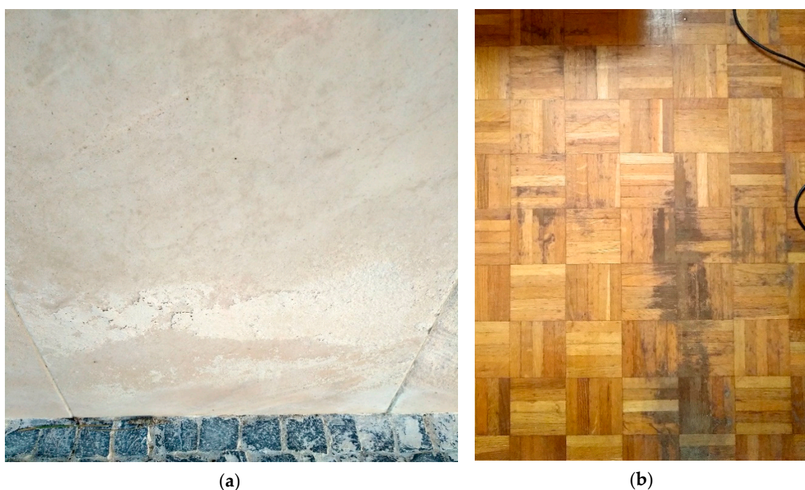
Figure 8. Signs of use of unprescribed, inadequate, incompatible, low-quality, non-certified and/or non-approved materials: (a) in a natural stone cladding in a maritime environment; (b) in a wood flooring.
