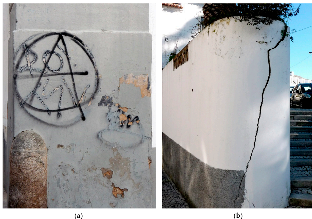
Figure 2. Examples of defects in the building envelope: (a) graffiti associated with vandalism and use and maintenance errors; (b) cracked wall due to mechanical actions.
