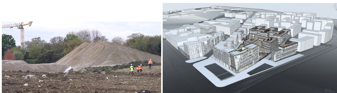
Figure 2. (Left): LaVallée: a 500 m × 400 m urban district under construction at present (2020). (Right): digital models of the buildings to be built. Credits: Atelier M3, Arcadis, SEMOP Châtenay-Malabry Parc-Centrale.
