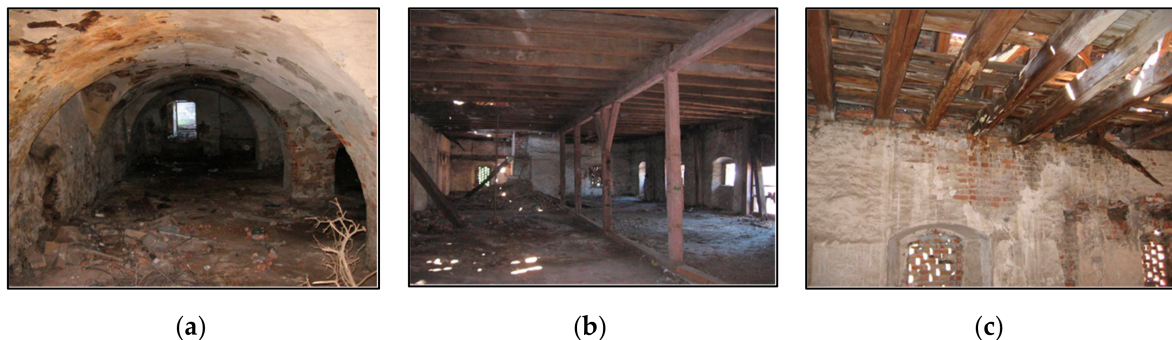
Figure 6. Granary building—cellar (a), first floor (b), second floor (c). (a) Moisture of vaults and basement pillars due to the lack of horizontal and vertical insulation. (b) First floor aboveground. (c) Damaged ends of floor beams in places where they rest on perimeter walls on the south side.
