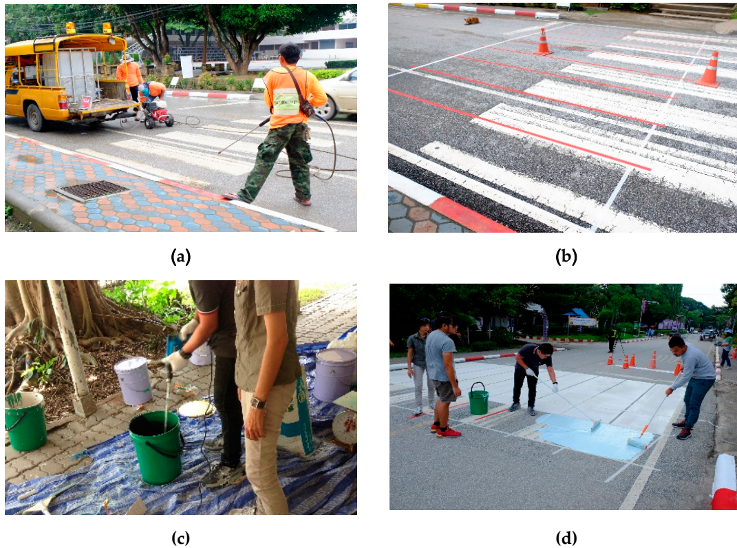
Figure 7. Installation of 3DPK crossing: (a) Removing existing zebra crossing paint, (b) road sketching before paint, (c) mixing materials, and (d) applying new paint.
