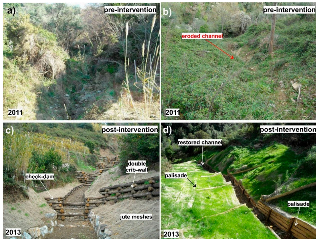
Figure 8. Representative examples of stream channel stabilization and hydraulic bioengineering works: channel conditions pre-intervention (a,b) and post-intervention; (c,d) (photos courtesy of Monterosso al Mare Municipality Administration).
