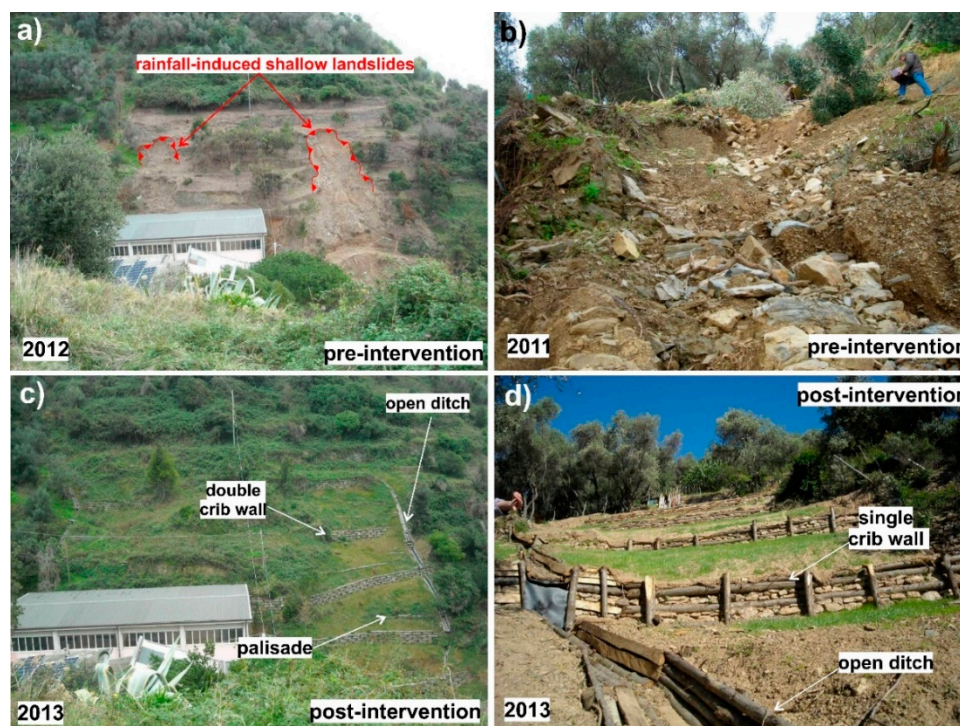
Figure 7. Representative examples of slope stabilization and landslide mitigation bioengineering works: slope conditions pre-intervention (a,b) and post-intervention (c,d) (photos courtesy of Monterosso al Mare Municipality Administration).
