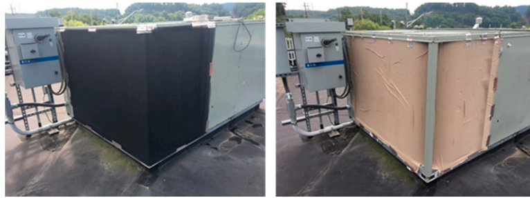
Figure 14. Fabric installation for condenser fouling test (left: 28% airflow reduction, right: 58% airflow reduction).
