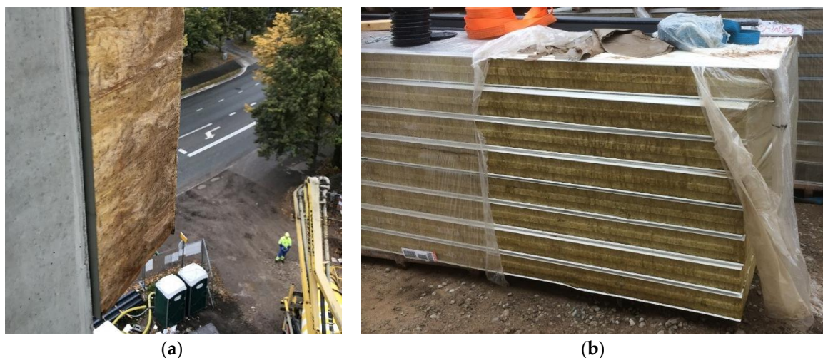
Figure 1. Sandwich panel insulating core exposed to outside environment during construction (a) and storage (b). Photos taken by the authors.
