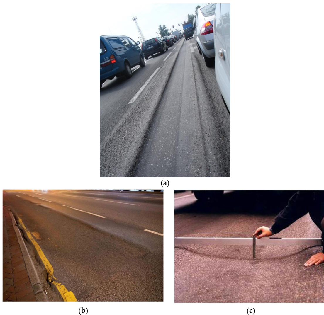
Figure 5. Rutting in asphalt pavements, adapted from (a) [69], (b) [70], and (c) [71].
