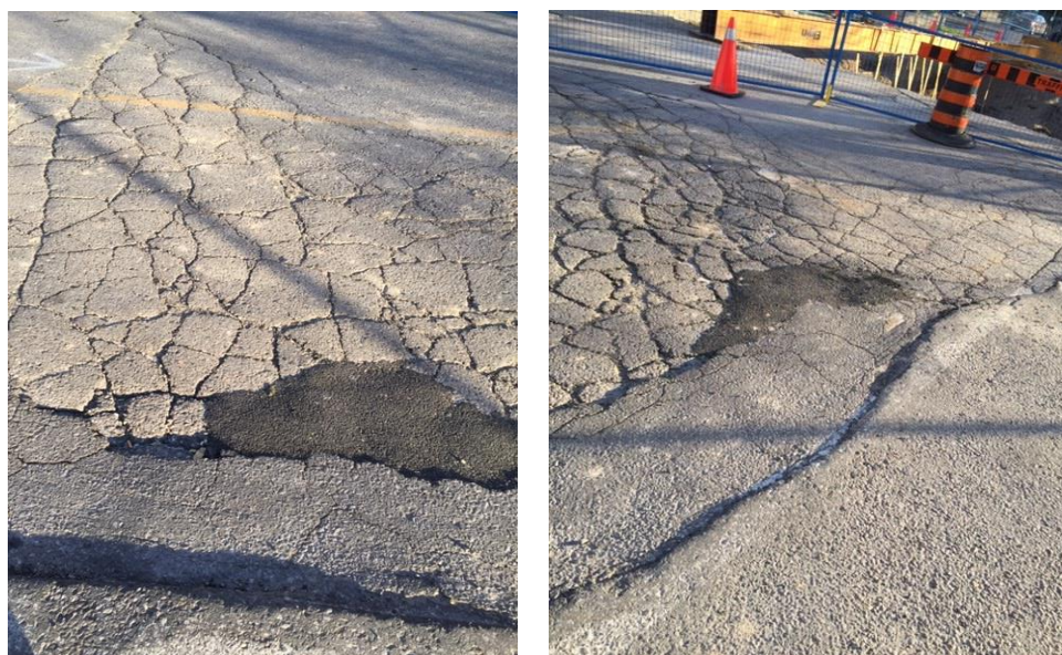
Figure 4. Fatigue cracking in asphalt pavements.
