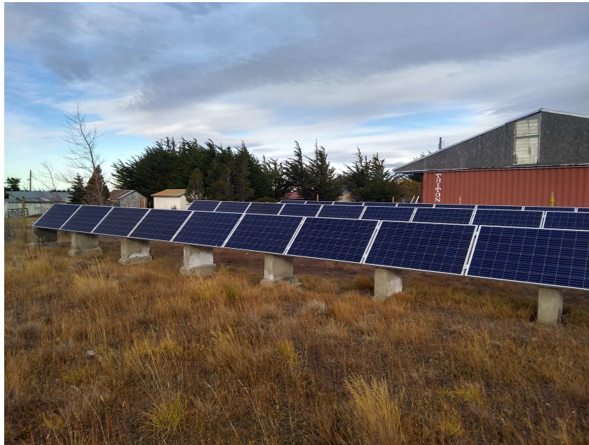
Figure 2. Photo of the installed 8.2 kW grid-connected photovoltaic system in Punta Arenas.
