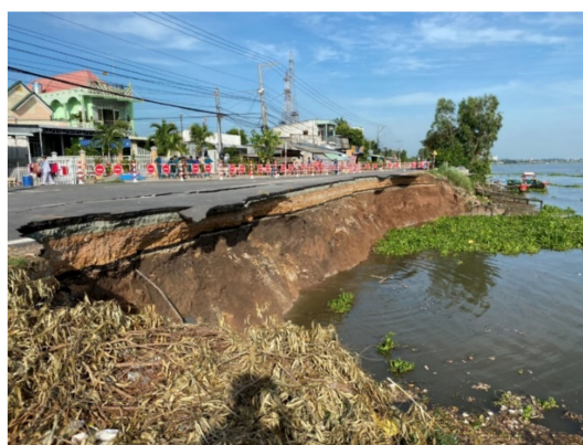
Figure 13. Section of National Highway in An Giang eroded into the Hau River, August 2019 (Source: Author Anh).
