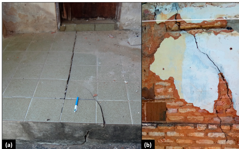
Figure 17. (a) Cracks in the floors; (b) Vertical, horizontal, and diagonal cracks in the masonry of residences in the study area.4. Discussion and Conclusions.
