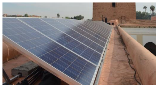
Figure 9. The installed PV panels in Koutoubia Mosque.
