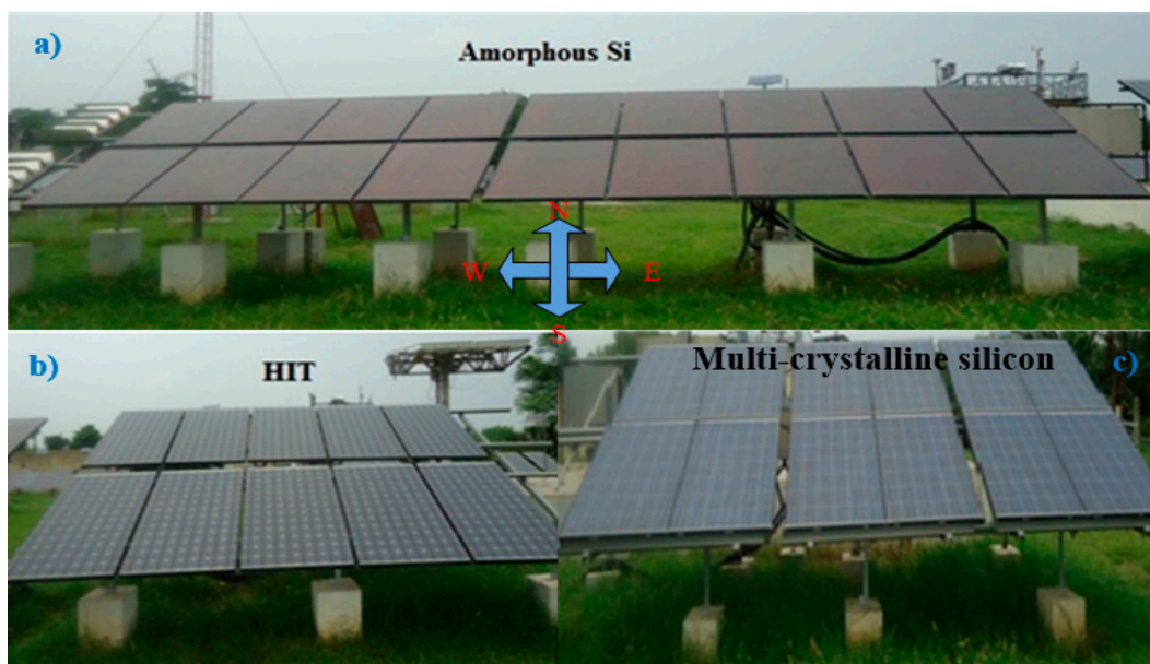
Figure 1. Experimental photovoltaic test facility at NISE, Gurgaon, India: (a). 1.2 kW Amorphous Si PV system; (b). 1.68 kW HIT PV system; (c). 1.6 kW Multi-crystalline silicon PV system.
