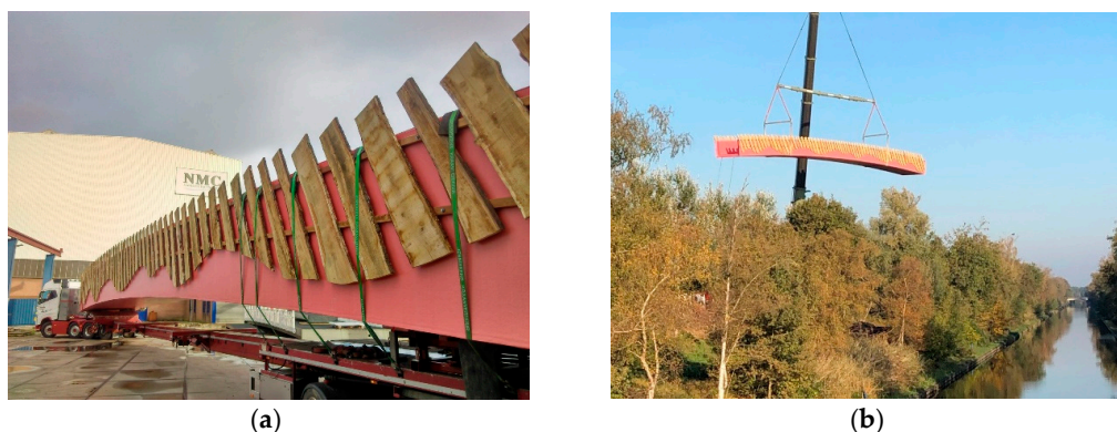
Figure 7. A uni-mold wildlife overpass with dimension of 36 m × 3.5 m in Eindhoven, The Netherlands. (a) The bridge was shipped on the back of a truck in one piece after manufacturing. (b) The single bridge span weighs 29 tons and was installed within a few hours using a single crane. Photo credits FiberCore Europe.
