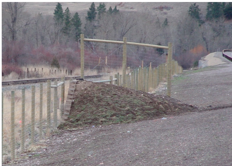
Figure 10. Wildlife jump-out and exclusion fencing along US Highway 93, Montana, USA. These structures are used to allow animals to jump down to the safe side of the fence and remove animals from the right-of-way. The wood elements in jump-outs and fencing can be replaced with recycled plastic FRP materials to better withstand the environmental elements and have a longer life cycle. Photo credit: Rob Ament.
