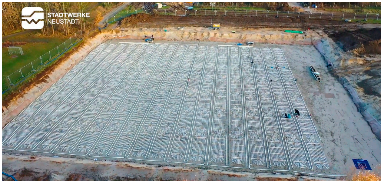
Figure 7. Aerial view of the installation of the approx. 3000 m 2 large-scale geothermal collector system below the rainwater retention basin in Neustadt am Rübenberge (Source: Stadtwerke Neustadt a. Rbge. GmbH, Neustadt am Rübenberge, Germany).
