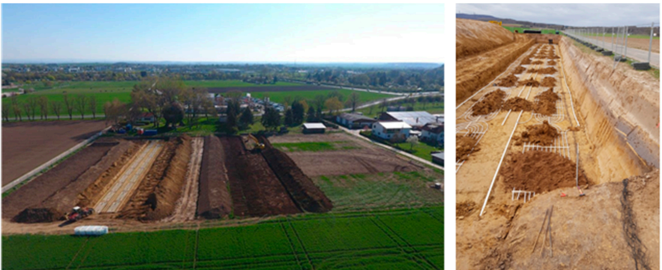
Figure 6. Construction site of the multilayer collector system in Bad Nauheim (Source: Steinhäuser GmbH & Co. KG, Bischberg, Germany).
