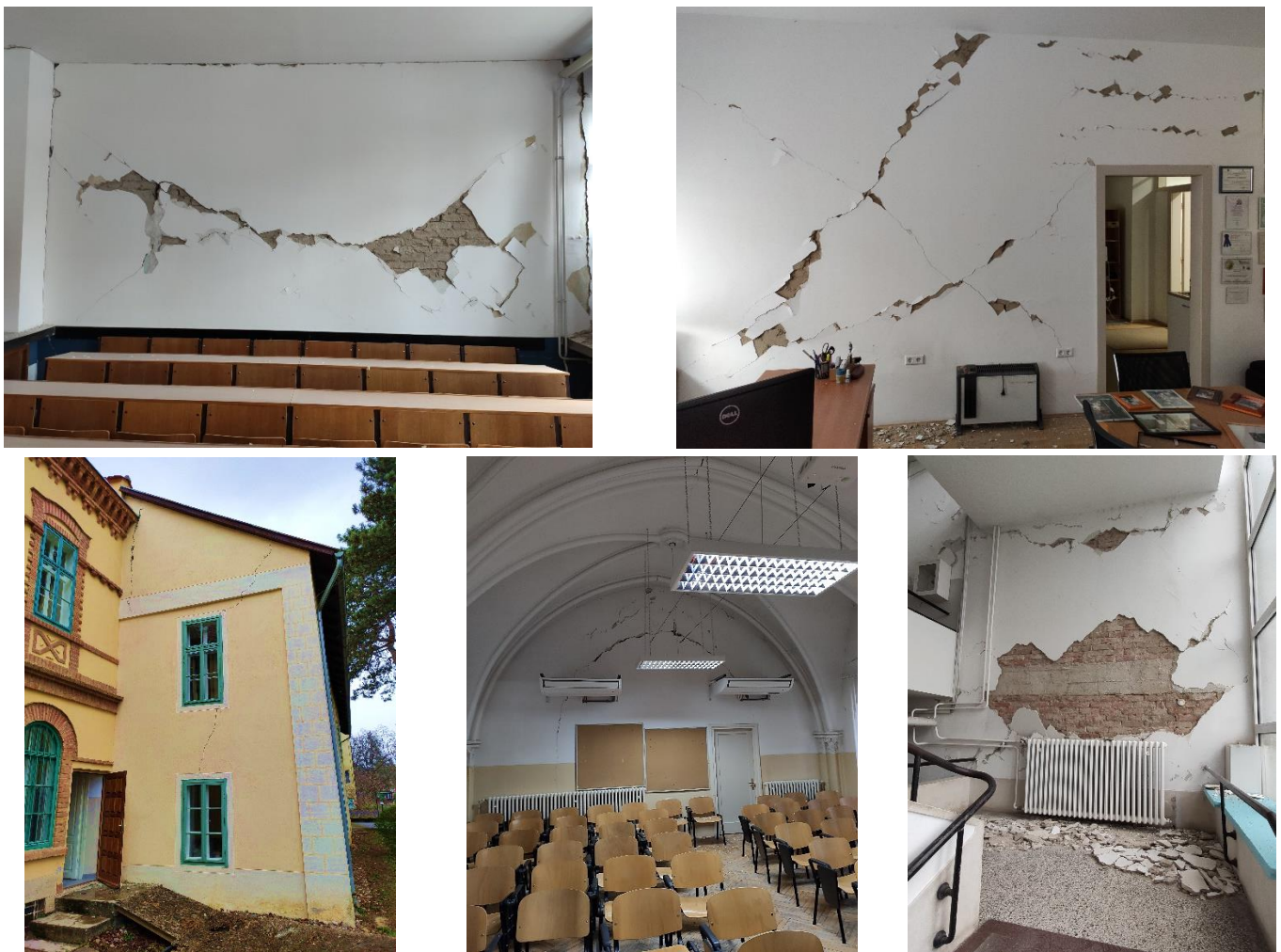
Figure 1. Typical damage to educational buildings after the Zagreb earthquake (photo credit: M. Stepinac).
