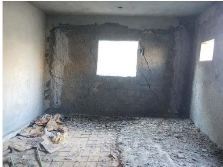
Figure 3. Excessive foundation settlement and cracking of the walls of a two-story house built on sabkha soil in the Eastern Province of Saudi Arabia.
