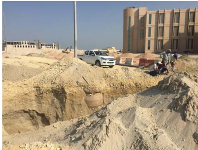
Figure 4. Very loose, poorly graded, and untreated subgrade stratum underlying relatively well graded, higher quality, and compacted sub-base and base courses. The resources and time utilized on the sub-base and base courses will be in vain once the poor subgrade strata settle under applied loads and varying degrees of saturation.
