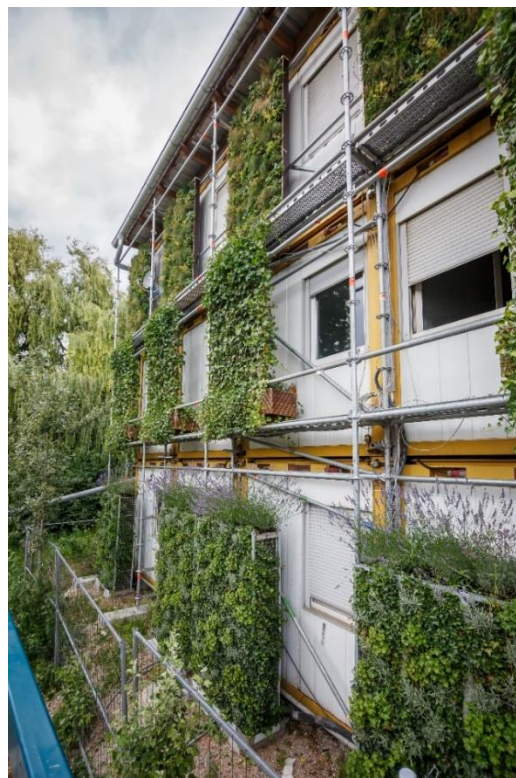
Figure 11. Three different systems of vertical greening were installed to investigate differences in performance. A scaffolding supports the plant boxes of the upper floors. Photo: Julian Rettig.
