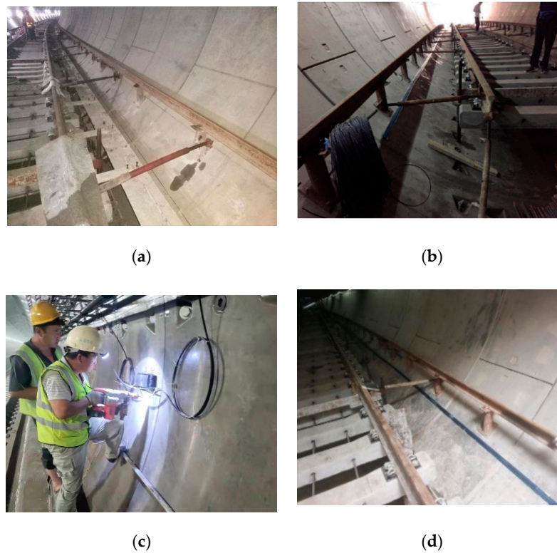
Figure 11. Construction photographs showing the optical fiber placement: (a) Inside the tunnel; (b) Pasting optical fiber sensors; (c) Construction; (d) After pasting the optical fiber.
