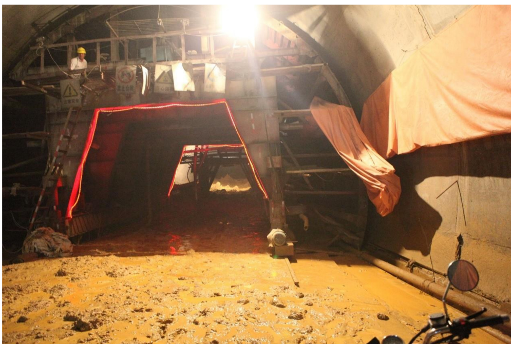
Figure 3. Water and mud inrush in the left tunnel for the second time.
