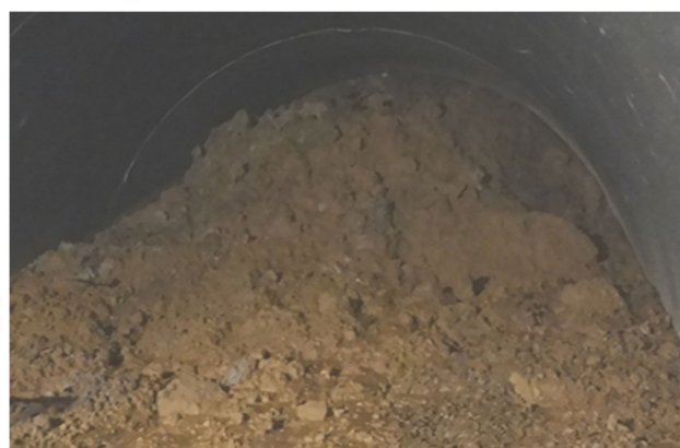
Figure 5. Inrush in right tunnel for the second time.
