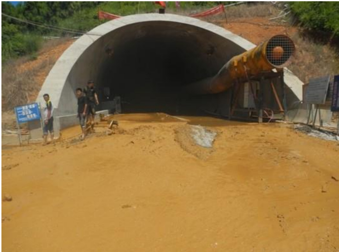
Figure 4. Water and mud inrush in left tunnel at third time.
