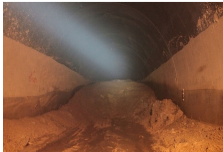
Figure 7. Inrush in right tunnel at sixth time.
