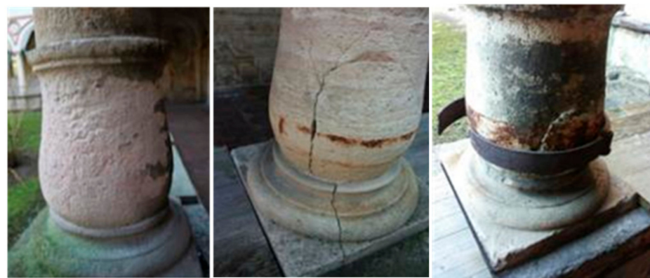
Figure 6. Degradation in the cloister's columns due to gypsum neogenesis with the presence of cracks in the columns' bulbs.
