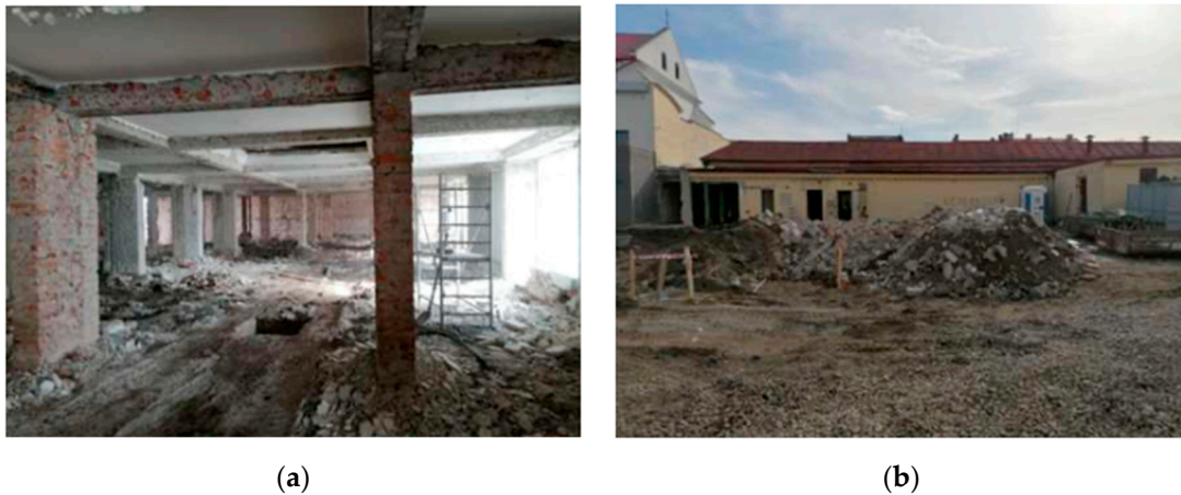
Figure 2. Demolition works (a) the interior of the building; (b) exterior of the building.
