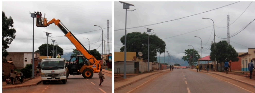
Figure 2. Foundation, installation, and start-up of a PV lighting installation in Cumbia, Angola. Aesthetic differences between ASL (left of the road) and AC grid aerial wires (right of the road).
