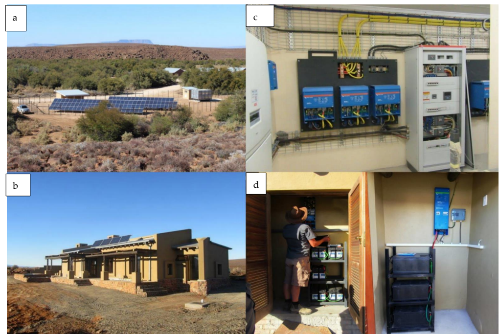
Figure 8. Example of a solar renewable system used in (a) TKNP Waaikop staff village and (b) TKNP's Elandsberg rest camp with solar panels installed on the roof. Battery and inverters installed and stored in a closet attached to the building on (c,d).
