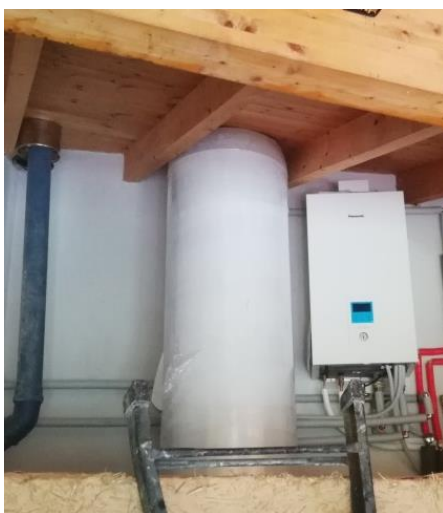
(a) Hot water tank
