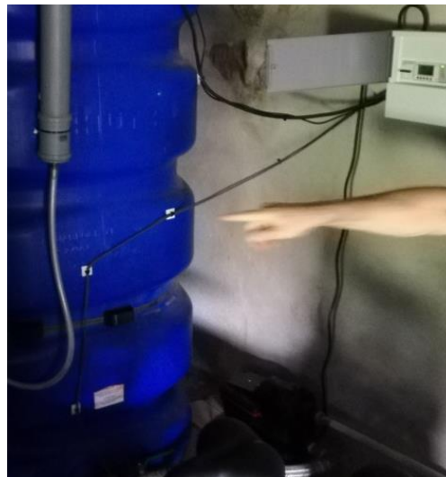
(b) Rainwater storage
