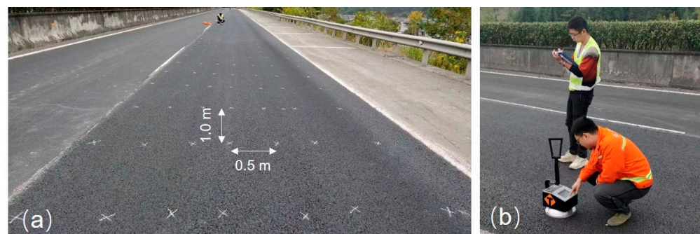
Figure 6. Field compactness test of a pavement section: (a) the arrangement of test points; (b) the field test on compactness of pavement using a non-nuclear densitometer.
