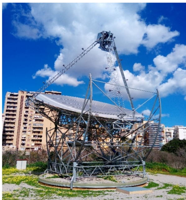
Figure 3. Dish-Stirling plant installed at the university campus of Palermo.
