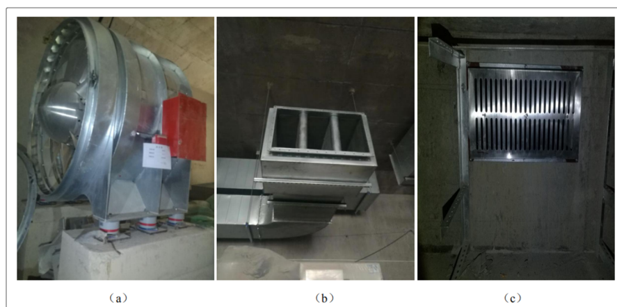
Figure 2. On-site investigation: (a) tunnel ventilation fan, (b) smoke exhaust pipe and muffler, and (c) rail bottom air duct.
