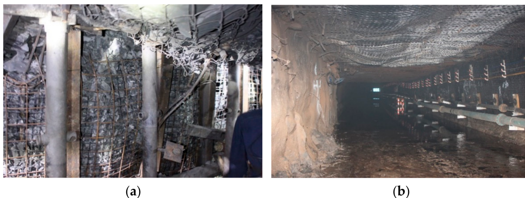
Figure 14. Engineering application. (a) The effect of roof caving. (b) Gob-side entry retaining by roof cutting.
