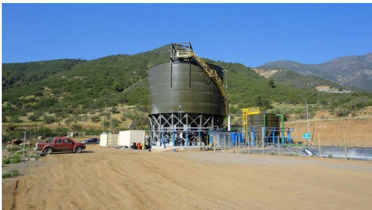
Figure 5. Tailings Deep Cone Thickener in Las Cenizas Mine—Chile.
