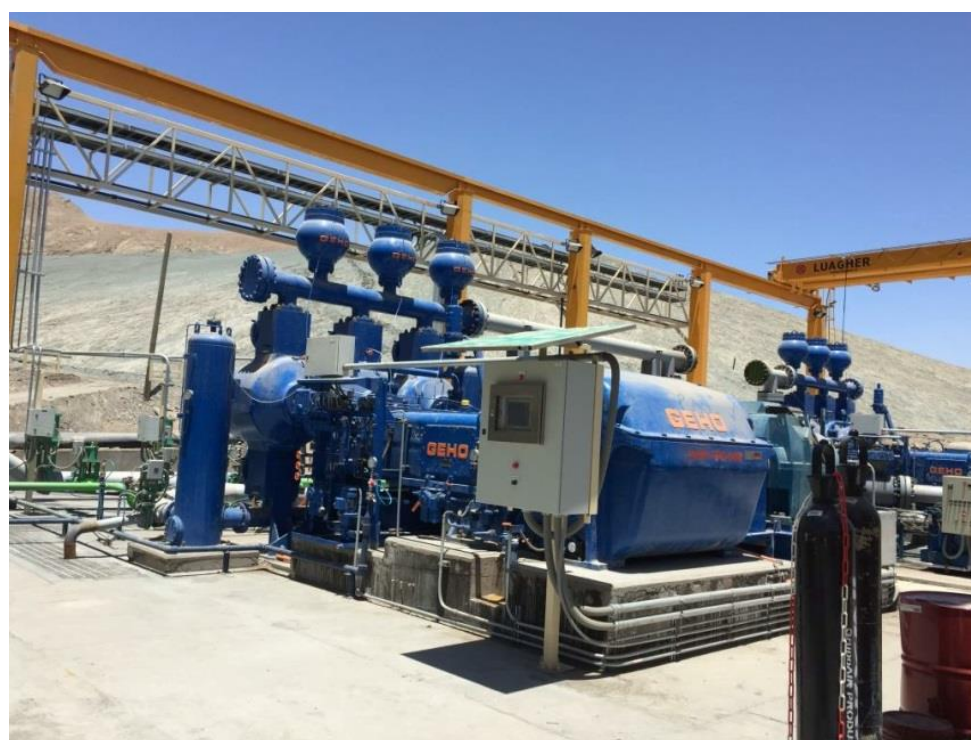
Figure 41. Coemin Positive Displacement Pump Station.
