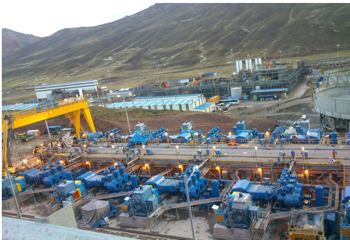
Figure 8. Thickened tailings positive displacement pump station—Toromocho Mining Project Peru.
