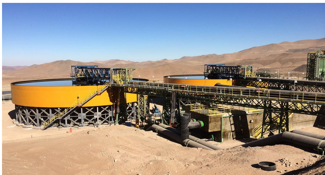
Figure 4. Tailings High Density Thickeners in Cerro Negro Norte Mine—Chile.
