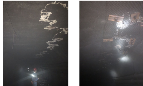
Figure 3. Ground pressure appearance of the surrounding rock of the main roadway.
