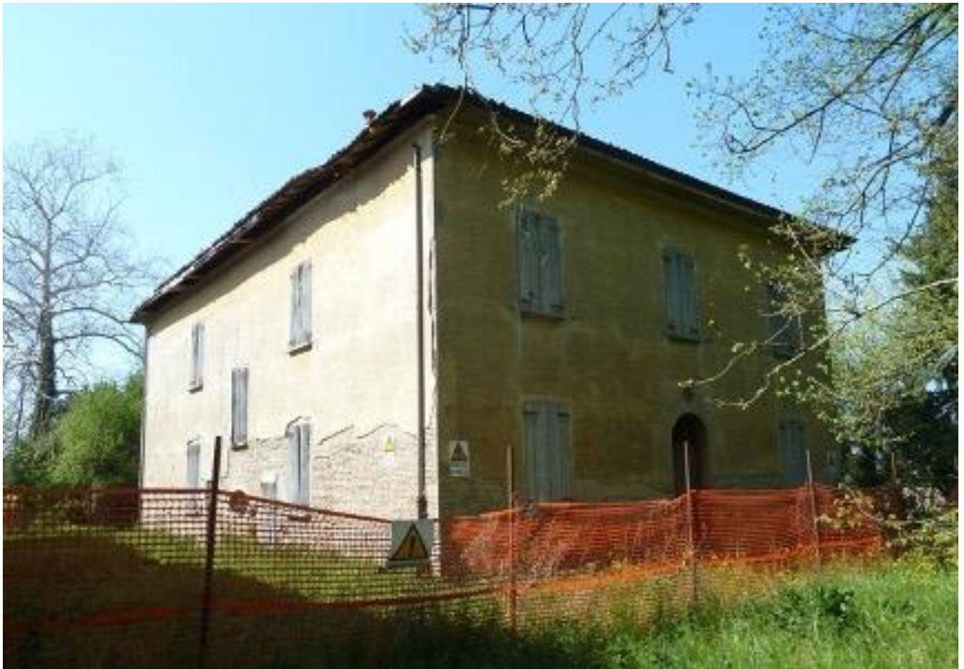
Figure 2. External view of the villa with load-bearing masonry walls in solid bricks (© 2020, Fondazione Carisbo).
