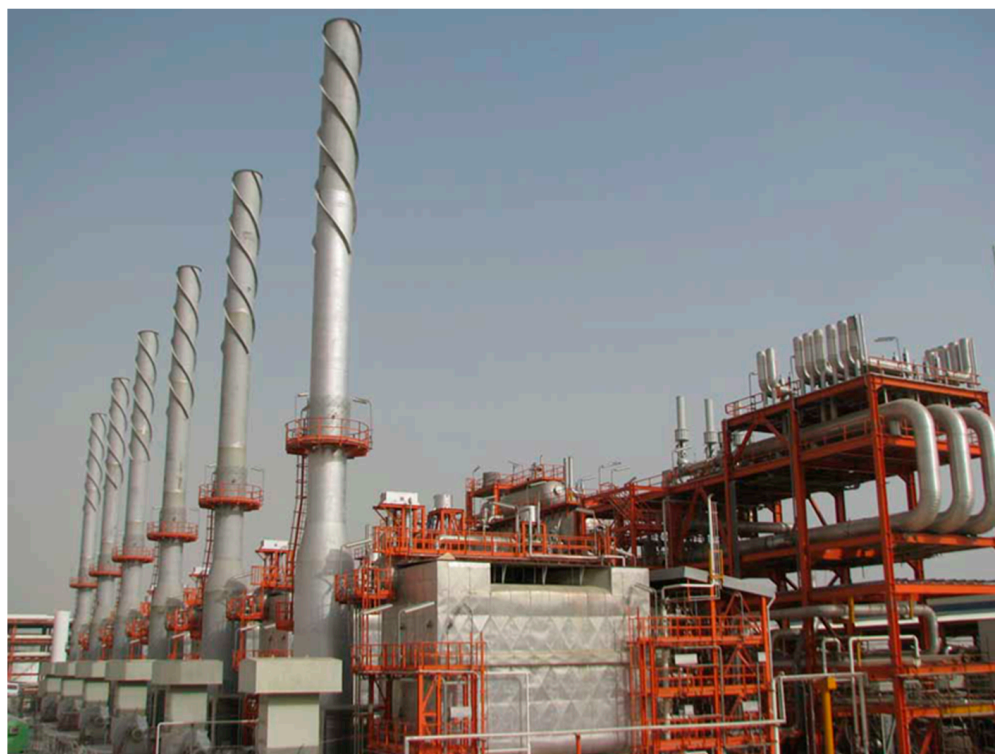
Figure 1. Boilers in the fourth refinery of the South Pars Gas Complex.
