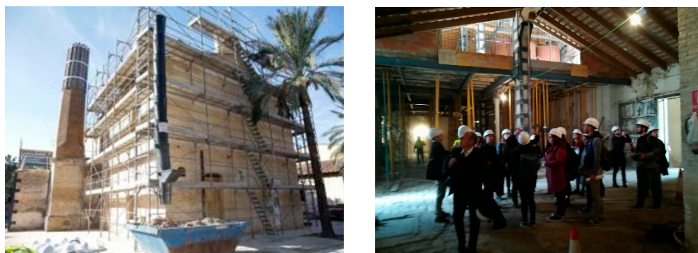
Figure 1. The Aceitera de Marxalenes during the restoration works. On the left : an external view of the chimney; On the right : internal view of the productive open space at ground level.
