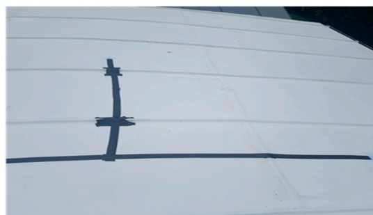
Sensor attached to the cool roof surface
