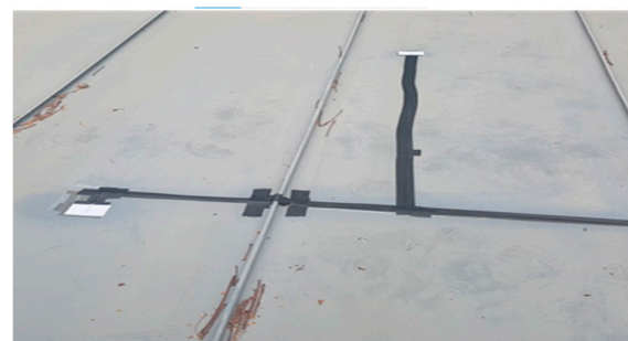
Sensor attached to the conventional roof surface
