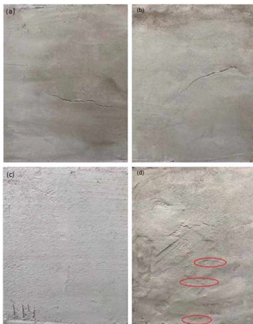
Figure 7. Visualization of cracks presence (red circle). Mixtures: (a) R01, (b) R02, (c) R03, (d) Hydrated Lime.
