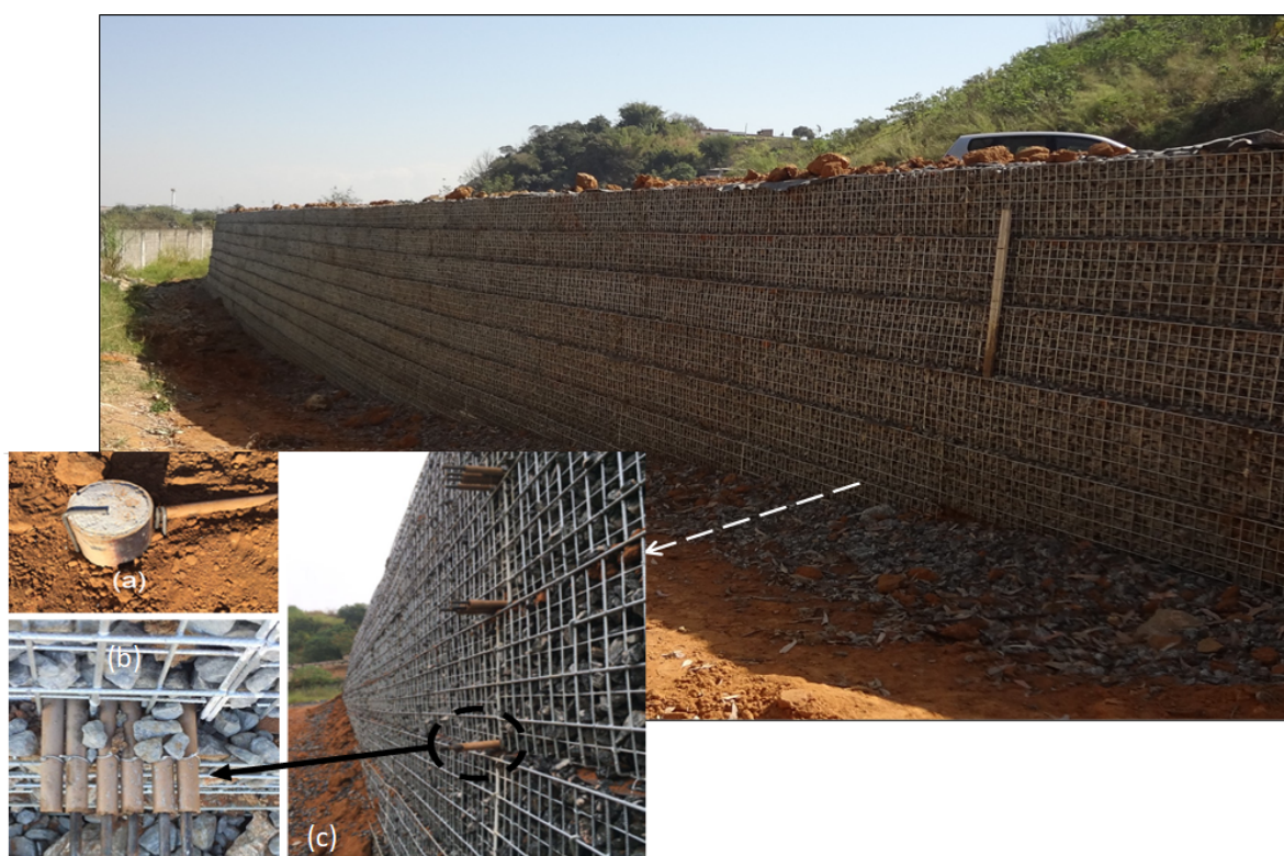
Figure 1. Overall view of the instrumented GRSW during construction: (a) installation of the reference bar for relative internal displacements; (b) view of the end of the extensometers used for relative displacement measurements; (c) view of the instrumented layers.
