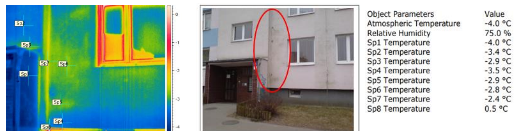
Figure 5. Biodegradation of the facade at the point of expansion of a panel apartment building and thermographic determination of temperature inhomogeneity [107,109].
