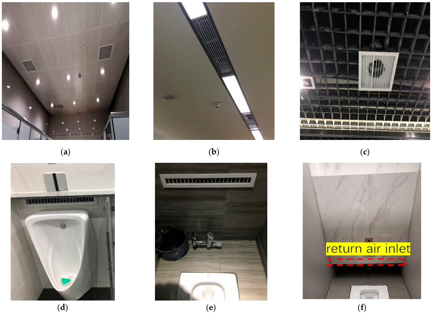
Figure 8. Ventilation system: (a) Square vent at the top (HZD); (b) Rectangle vent at the top (HZD(G)); (c) The fresh air outlet at the top (NJ); (d) Rectangle vent at bottom (NJ); (e) Rectangle vent at bottom (0.8 m) (ZJ); (f) Rectangle vent at bottom (0.3 m) (HZD(G)).
