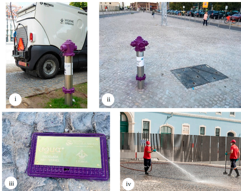
Figure 5. Water reuse hydrant network in downtown Lisbon. (i,ii) First water reuse hydrants installed in downtown Lisbon area; (iii) Water reuse ground hydrant in downtown Lisbon; (iv) Urban hygiene staff washing a street using treated wastewater in downtown Lisbon.
