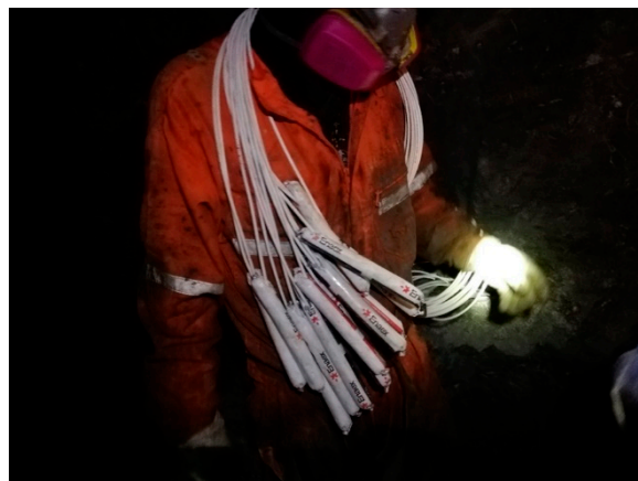
Figure 8. Explosives handling (incorrect and dangerous).
