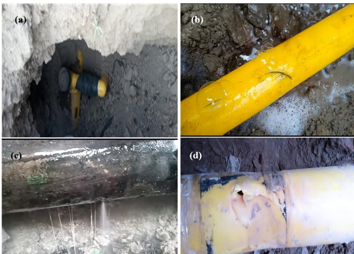
Figure 5. Underground gas leakage detections at (a) a 4-inch polyethylene main line with a 2-inch offtake line, (b) a 1.25-inch polyethylene feeder main line with two visible cuts, (c) a 4-inch mild steel pipeline, and (d) a 2-inch polyethylene line damaged by excavation activity.
