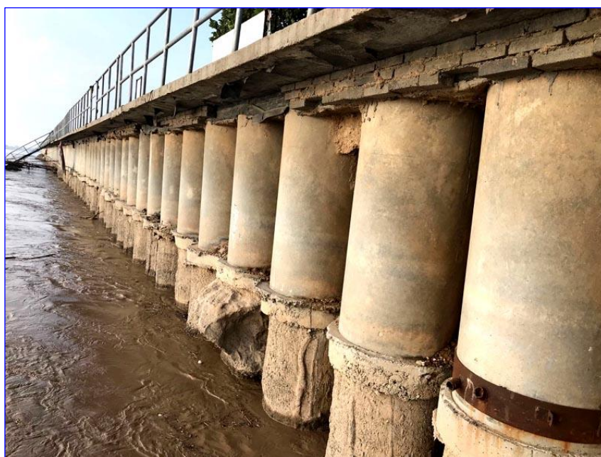
Figure 2. Piles along the riverbank of the Yellow River. Photo by Xiangzhou Xu, 15 July 2018.
