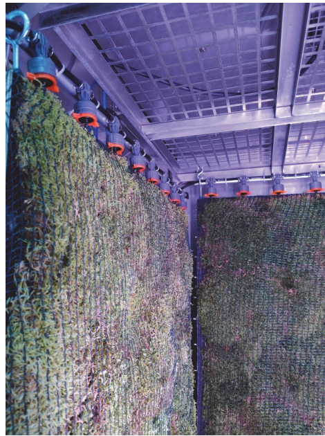
Figure 6. Fixed spray irrigation at the upper end of the panels.
