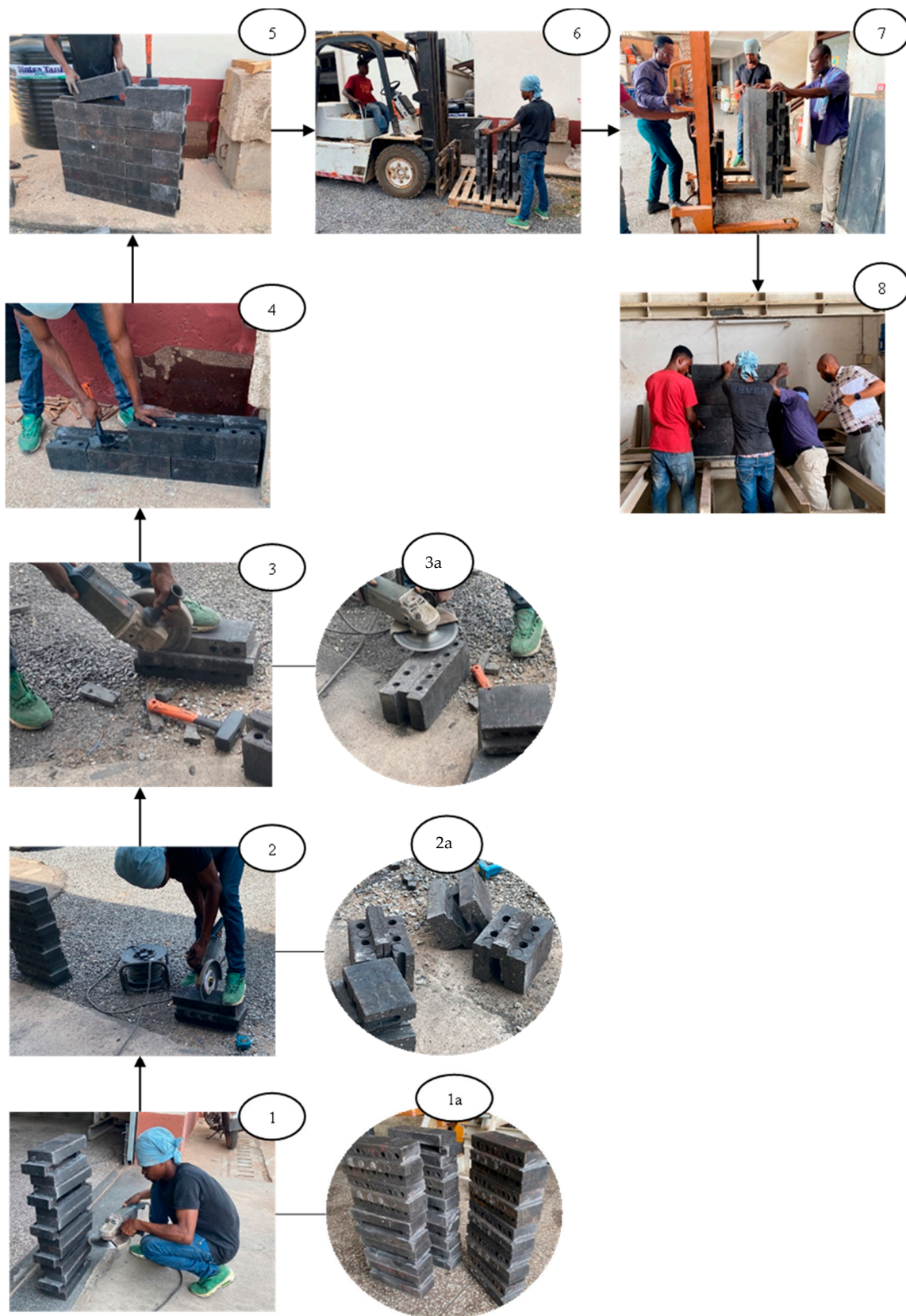
Figure 5. Fabrication process of the plastic-bonded sand interlocking block wall. The excess block protrusions are first removed. Half blocks are then cut from the stretcher blocks. The base course is then laid by hammering the block protrusions into grooves of adjacent blocks before continuing with the subsequent courses.
