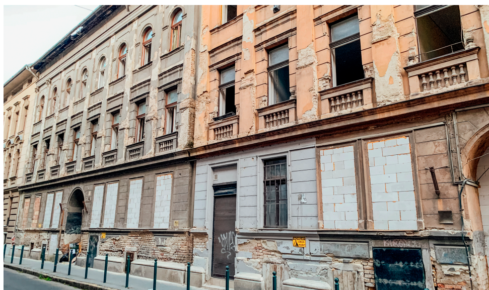
Figure 10. Structures at Viola Street vacated and isolated by the local municipality have languished for years, awaiting renovation efforts. Local residents were either compensated or relocated to alternative housing managed by the municipality while awaiting the completion of the construction works. However, this strategy intensifies challenges tied to urban gentrification, furthering the displacement of vulnerable populations to the city’s outskirts.
