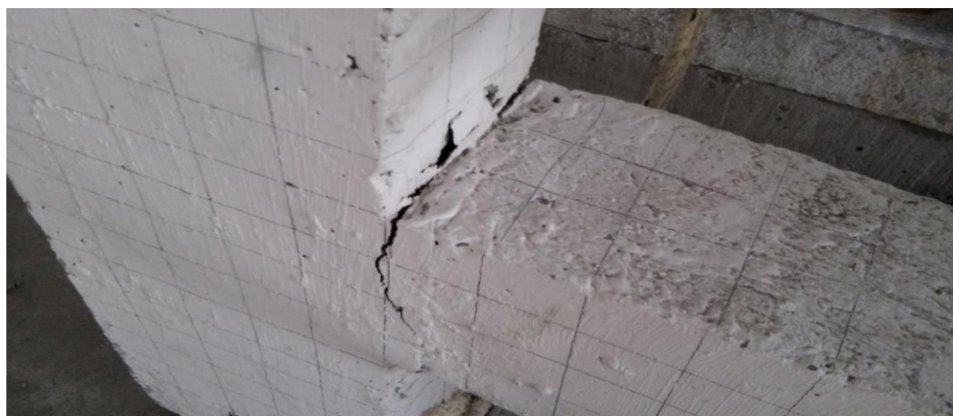
Figure 12. Initial cracks in the beam column joint.
