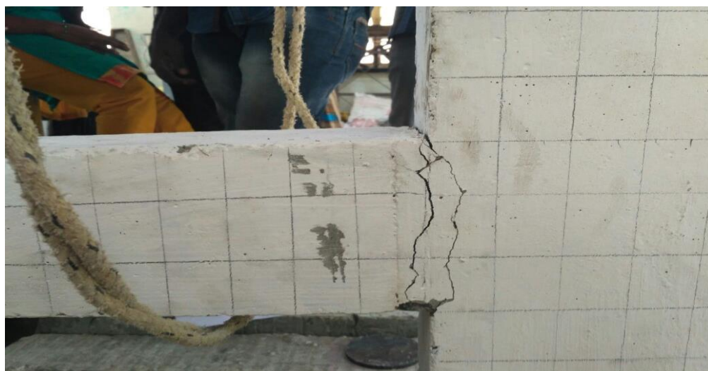
Figure 13. Failure mode of the beam column joint.
